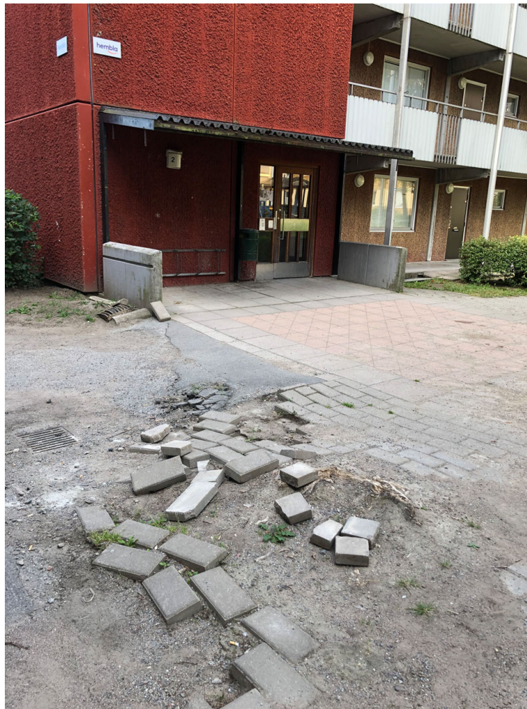
Figure 2: Maintenance issues on Nidarosgatan, Husby, May 2020 (source: authors)
